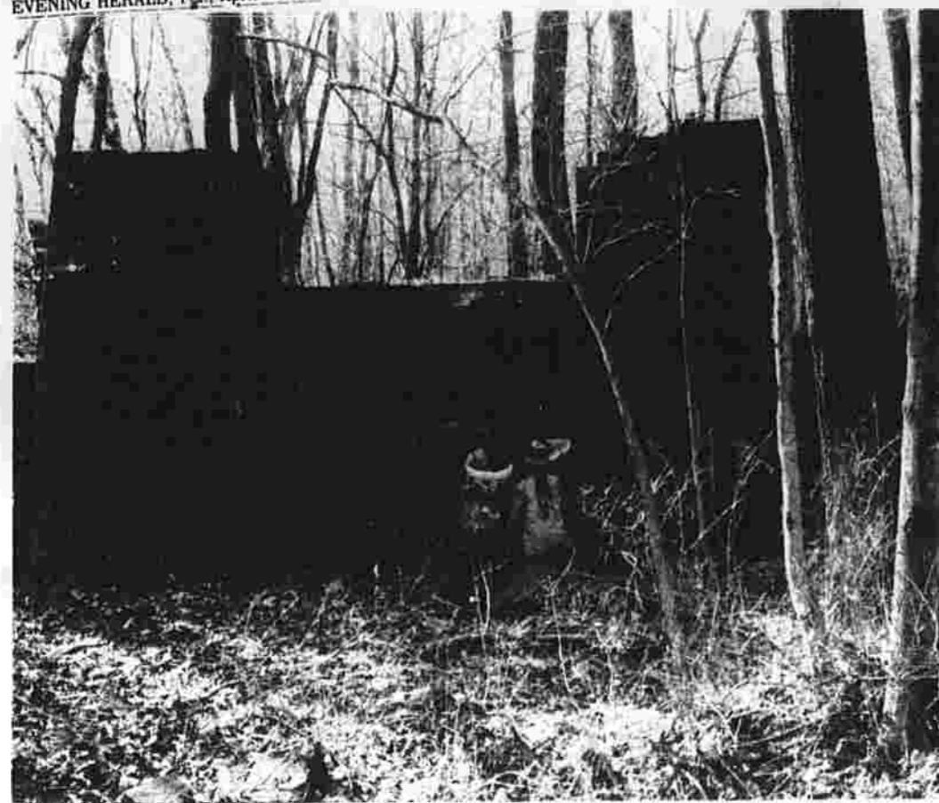
A dam built in 1869 is examined by hikers near the old Peter Adams Paper Mill through which one of the committee's four trails passes. The dam was part of a system of
